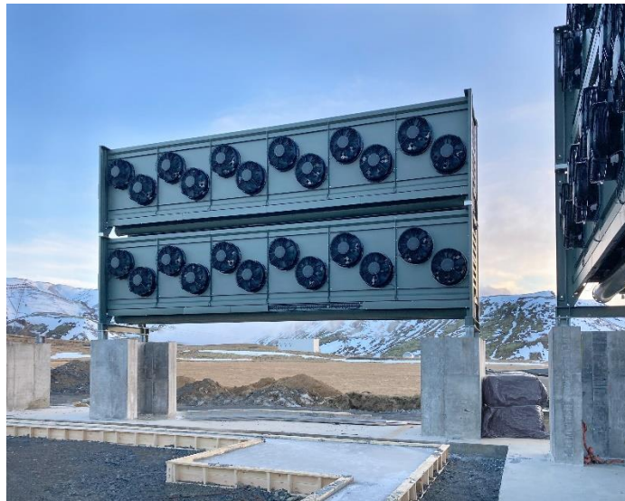
Climeworks direct air capture facility in Iceland
