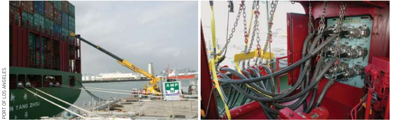
Left: A crane lifts the electrical plugs of the shore-side power system to a ship at the Port of Los Angeles. Right: A close-up of a ship's electrical "plug-in" to shore-side power at the Port of Los Angeles.
