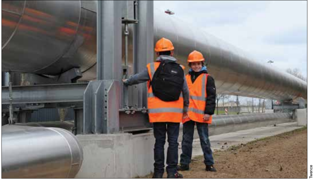
A pipeline transports steam produced by the Twence waste incinerator to the neighboring Akzo Nobel salt factory, which uses the steam to produce salt from a mine below the factory, avoiding the need to burn 40 million cubic meters of natural gas every year.
